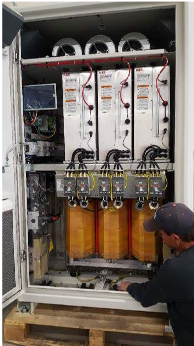
BATTERY ELECTRIC BUS CHARGING INSTALLATION
